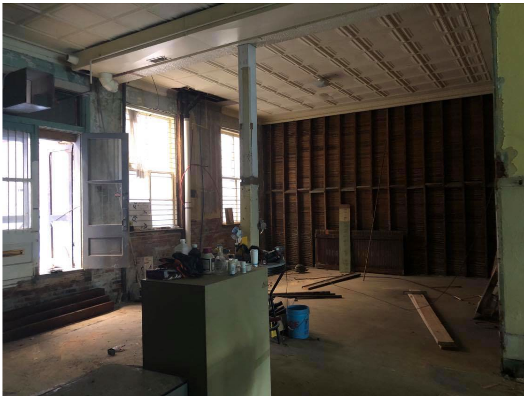
Figure 19: Interior of rear section of 217 Colorado Avenue storefront in January 2021 during ongoing renovation. (Mondello's Opera House Pizzeria/Facebook)
