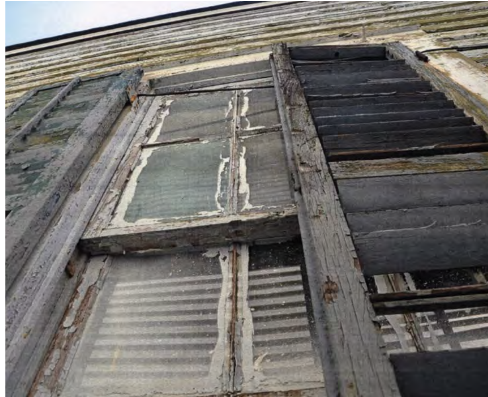
[11] Old and brittle glazing putty should be removed carefully before reputtying to keep window glazing weathertight.
