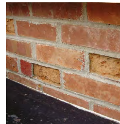
[2] Not Recommended: The use of inappropriate Portland cement mortar to repoint these soft 19th-century bricks has caused some of them to spall. Photo: Courtesy Nebraska State Historic Preservation Office.
