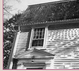
Left and center: City Hall, Saco, Maine (1855) Right: Edward Devotion House Brookline, Massachusetts (ca. 1680 frame; 1740)
