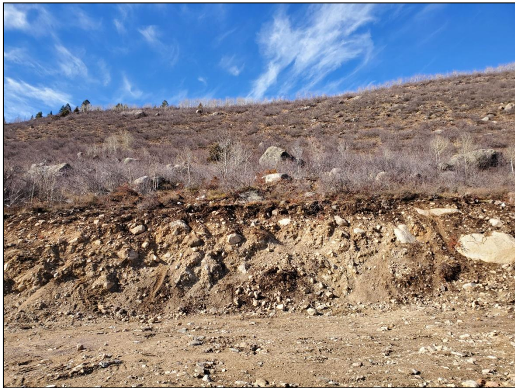
Overview of the tank location towards the already excavated wall (Roll 20-104, unaltered image 04, 11/22/2020)
