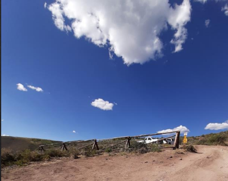
Assembling Buck N' Rail Fence at Metcalf Rd, preventing illegal snowmobile access
